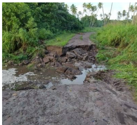
Figure 12g: Road collapse in Nabukelevu-i-ra Road in Kadavu, Eastern Division on the 4 th . Source: Fiji Roads Authority.
