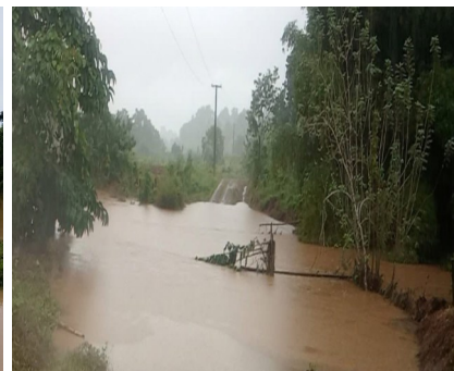
Figure 12c: Flooded road in Korovou, Central Division, on the 16 th . Source: Fiji Roads Authority.
