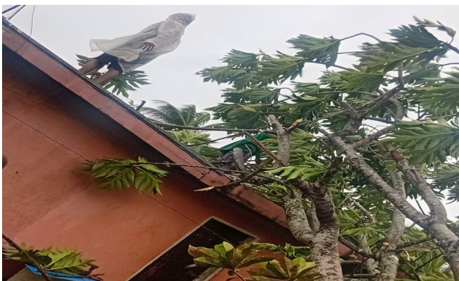
Figure 14r: Clearing of debris from roof of a home in Moala Village, Western Division. Source: Fiji Red Cross Society.
