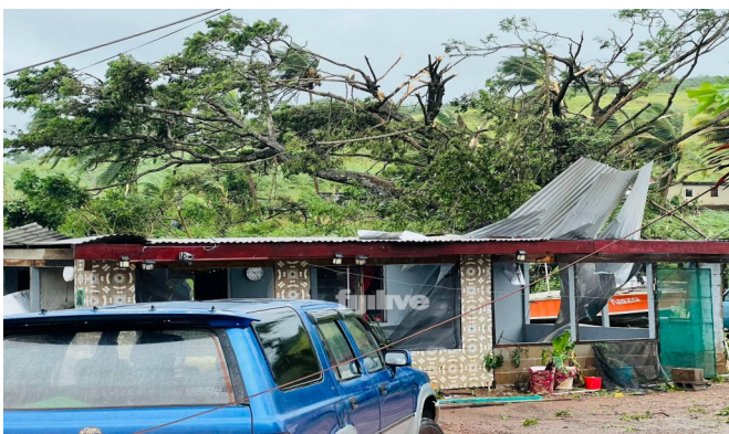
Figure 14t: Roof damage from strong winds to a house in Drasa, Lautoka, Western Division. Source: FijiLive.
