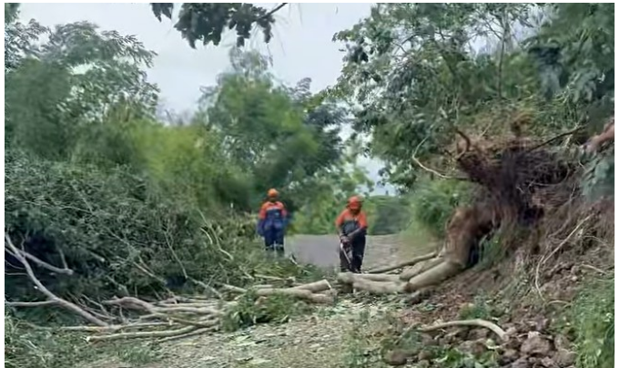
Figure 14h: Clean up operations of debris in the Western Division. Source: Bose Vavataga.
