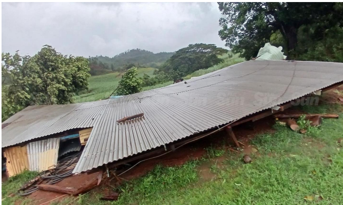
Figure 14i: A collapsed home in Lautoka, Western Division. Source: The Fiji Times.
