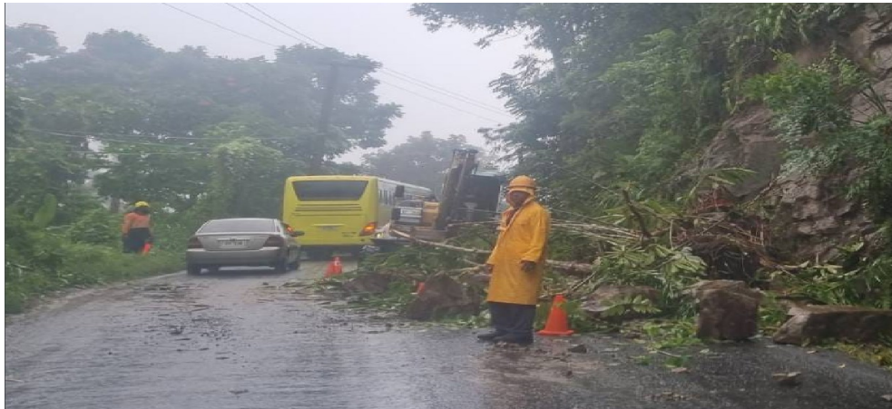
Figure 12: Massive rocks, soil and debris lying on the roadside due to the landslide on 27 th July, 2023. Source: Fiji Roads Authority
