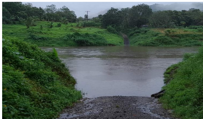
Figure 12t: Wainibuka crossing, Colata Cocoa Road on the 25 th . Source: Fiji Roads Authority.
