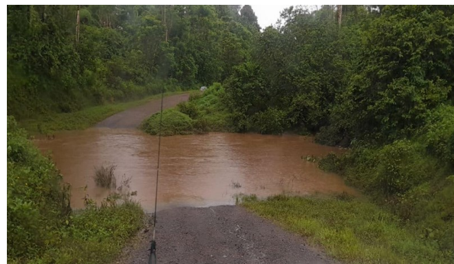
Figure 12l: Waidradra Crossing at Vatulili Road on the 21 st . Source: National Disaster Management Office.
