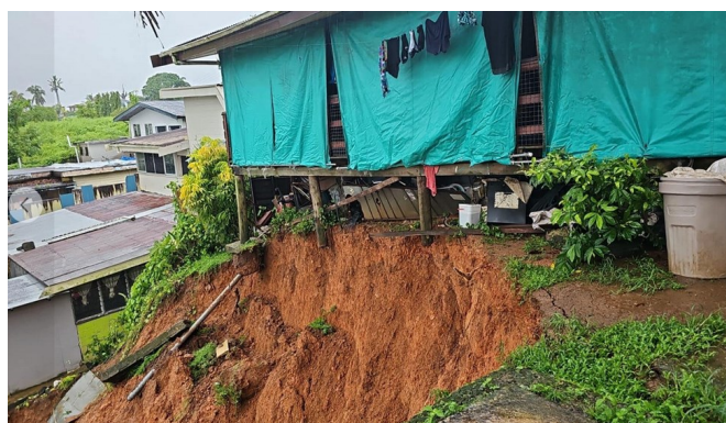
Figure 12j: Landslide at Kula Street in Samabula on the 20 th . Source: National Disaster Management Office.
