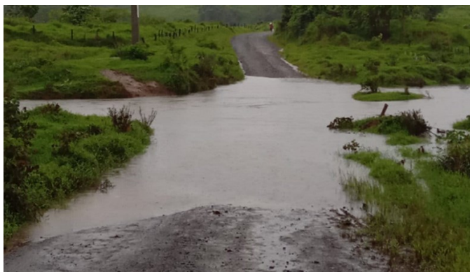
Figure 12s: Navulokani Road, Central Division on the 25 th . Source: Fiji Roads Authority.
