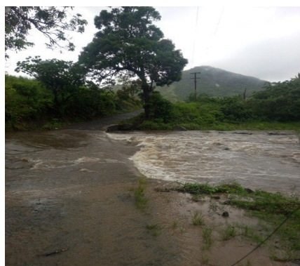
Figure 12b: Narara crossing flooding on the 24 th . Source: Fiji Roads Authority.
